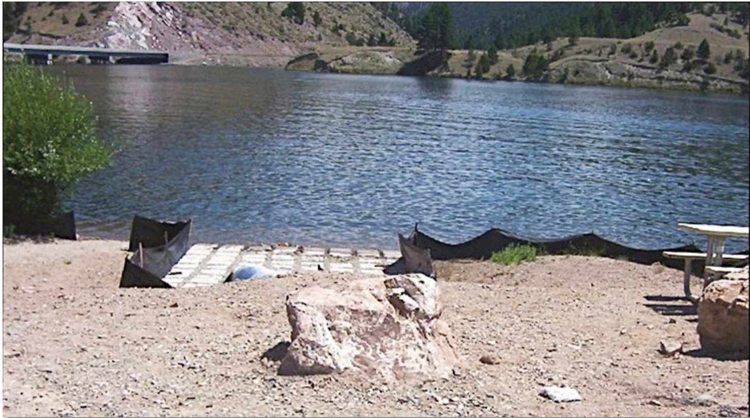
An articulated concrete launch helps to protect against the effects of erosion while providing paddlers with a separate access site from heavy boat traffic.
