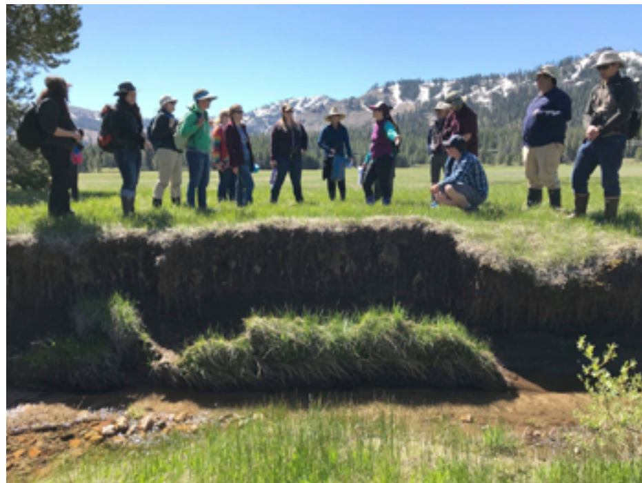
Active erosion in Castle Creek within Van Norden Meadow. Taken during a public tour in 2018, showing erosion after the 2017 Water Year. Credit: SYRCL
