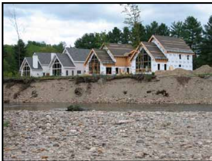
Development under construction along the West Branch of the Little River in Stowe, Vermont, above the 100 year floodplain elevation but within the meander belt area of a highly unstable reach. Projects like this, and the increasing expense of channelizing the river to protect riparian investments in town, led Stowe to be the first Vermont municipality to adopt an FEH zone to curtail further encroachment. Photo: Vermont Rivers Program
